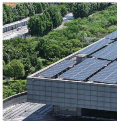
Anhui Tongling Enterprise and Institution PV Project
