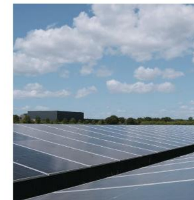
Netherlands Ground Power Station Project Project Capacity | 13.62MW
