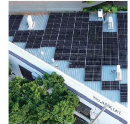
Australian Commercial Shop Rooftop Project Project Capacity | 30.71kW
