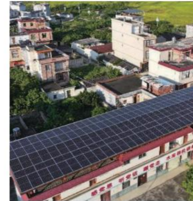
Guangxi Skyworth Xiaoyang Building PV Project Project Capacity | 199.8kW
