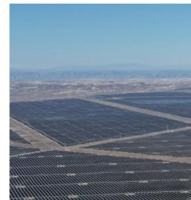
900,000 kilowatts Qinghai Gonghe PV Project Project Capacity | 900MW
